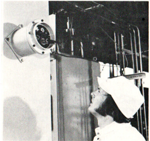
Installed gamma monitor and alarm.
