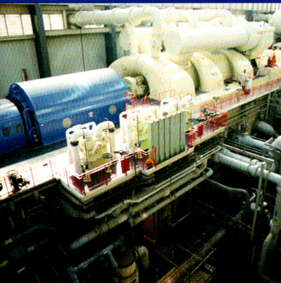
Oldbury power station turbine hall.
