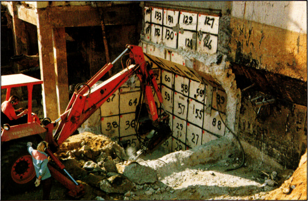
Figure 5. Standard or slightly modified demolition techniques can be used for many decommissioning operations. (Photo: Rockwell International)
