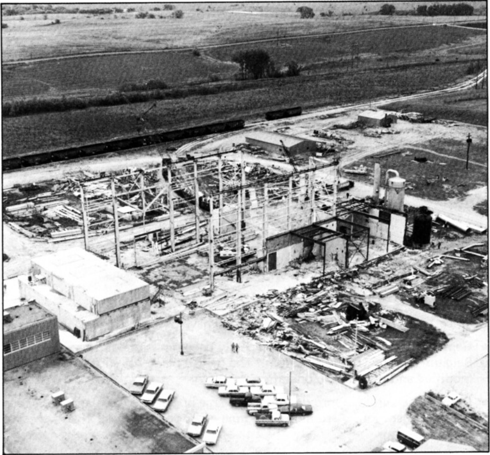
Figure 4. The Hallam reactor in the USA was decommissioned to Stage 2; the work is shown here nearing completion. (Photo: Rockwell International)
